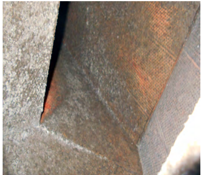
Example of white toxic mold hiding in the fiberglass lined AC supply plenum above the AC. Invisible unless the air handler is first removed. Not accessible to air duct cleaners.
