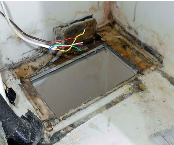
Example of black toxic mold hiding in AC closet. Invisible unless the air handler is first removed. Not accessible to air duct cleaners.
